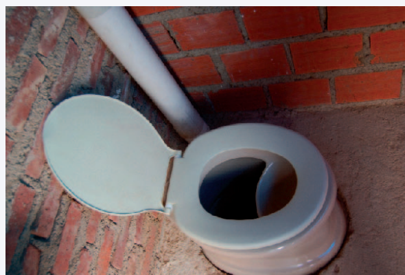
Figure 6. Interior of bathroom with urine diverting toilet
