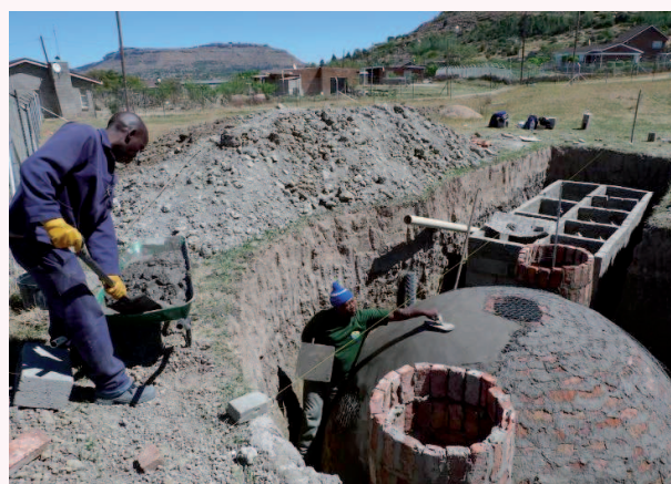
Figure 3: Approaching the final stage of construction: biogas digester and anaerobic baffled reactor before being covered with soil and installation of planted gravel filter will start
