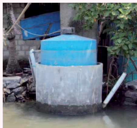
Figure 5: Biogas plant discharging directly into the backwaters
