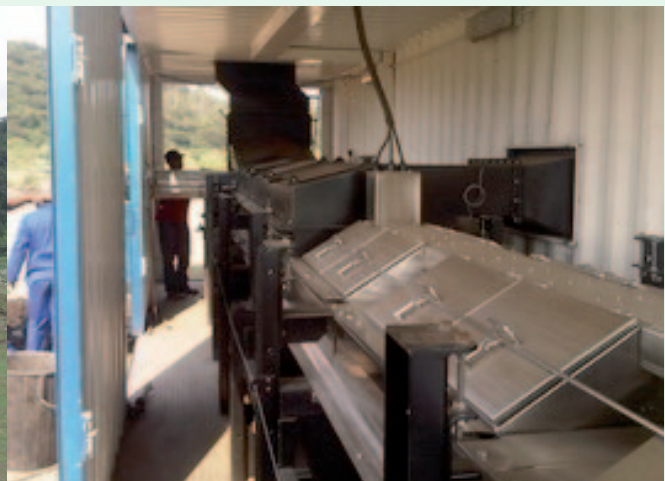
Figure 3 – The LaDePa machine inside the container.
