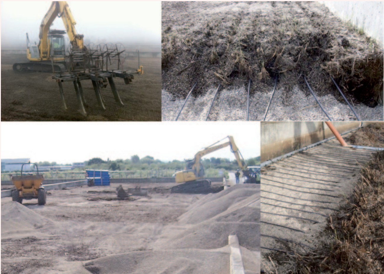
Figure 3: Retrofit of an aeration system into an existing treatment wetland at Mayfield Farm, UK.
