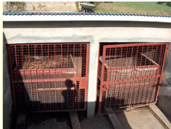
Figure 5: Filter baskets for pre-treatment of wastewater.
