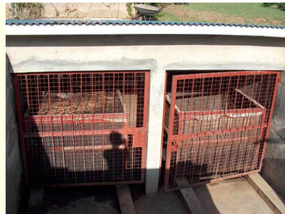
Figure 5: Filter baskets for pre-treatment of wastewater.
